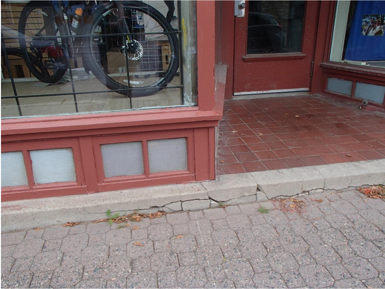
Photo: Cracked cement along front edge
