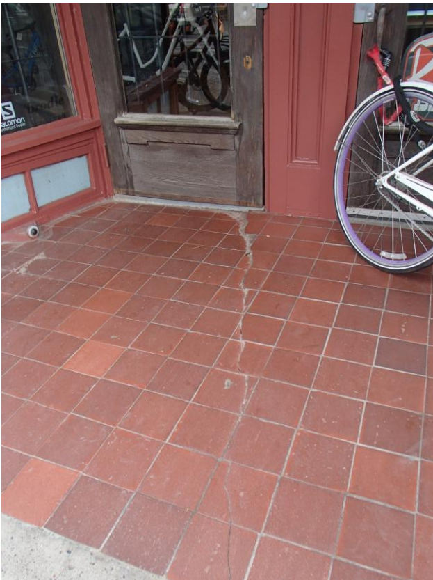
Photo: Crack in stone tiles outside entrance
