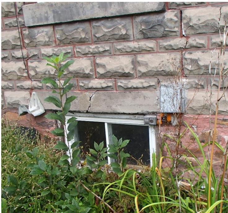
Photo: Concrete lintels on south side are cracked
