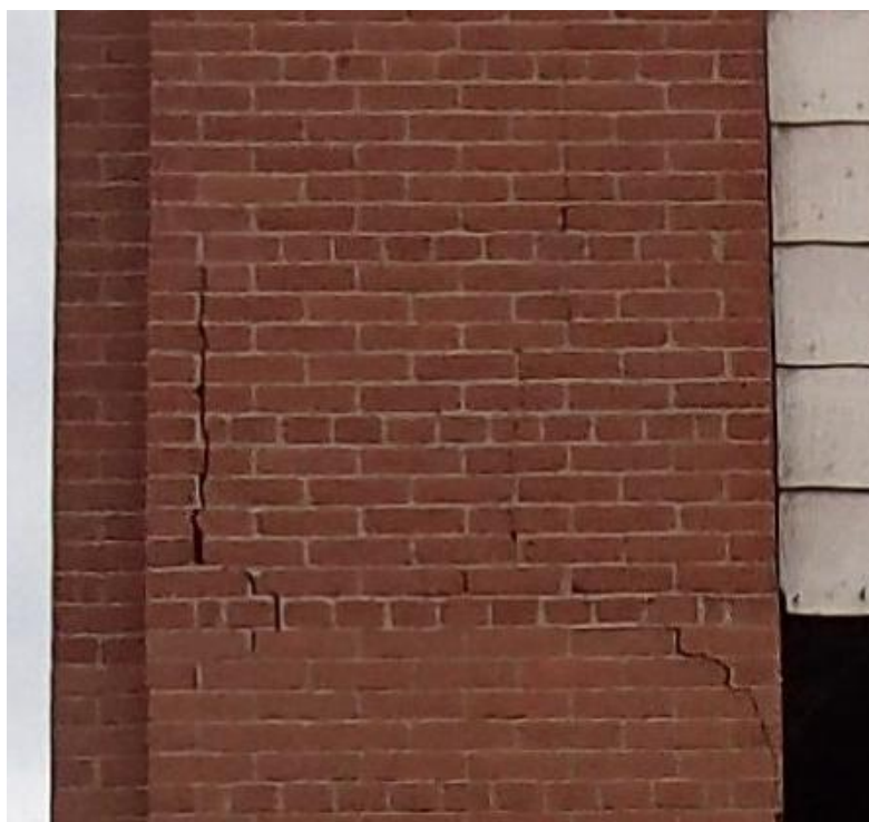
Photo: Close up of crack in brickwork – south side – second storey.
