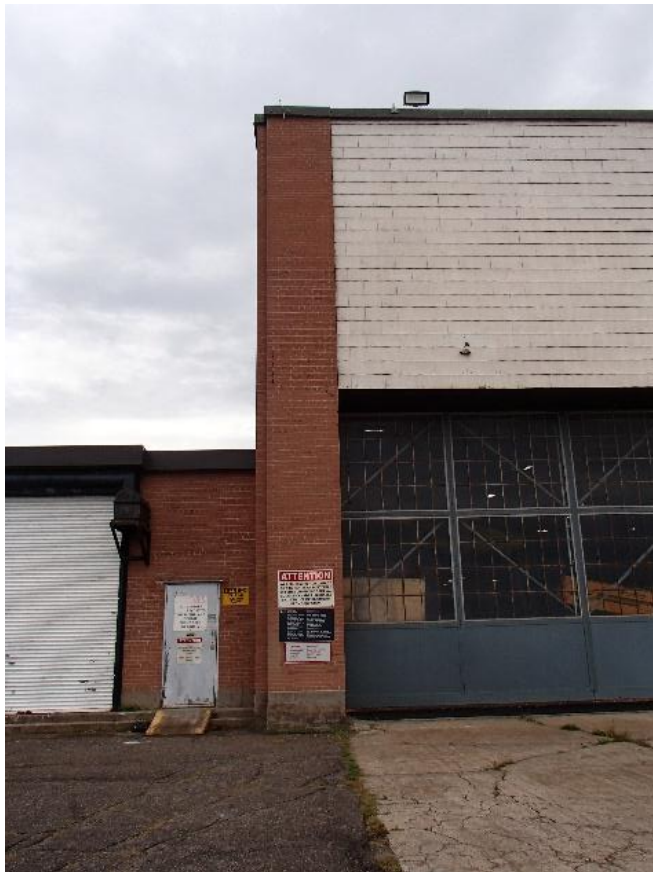
Photo: South side crack in brickwork
