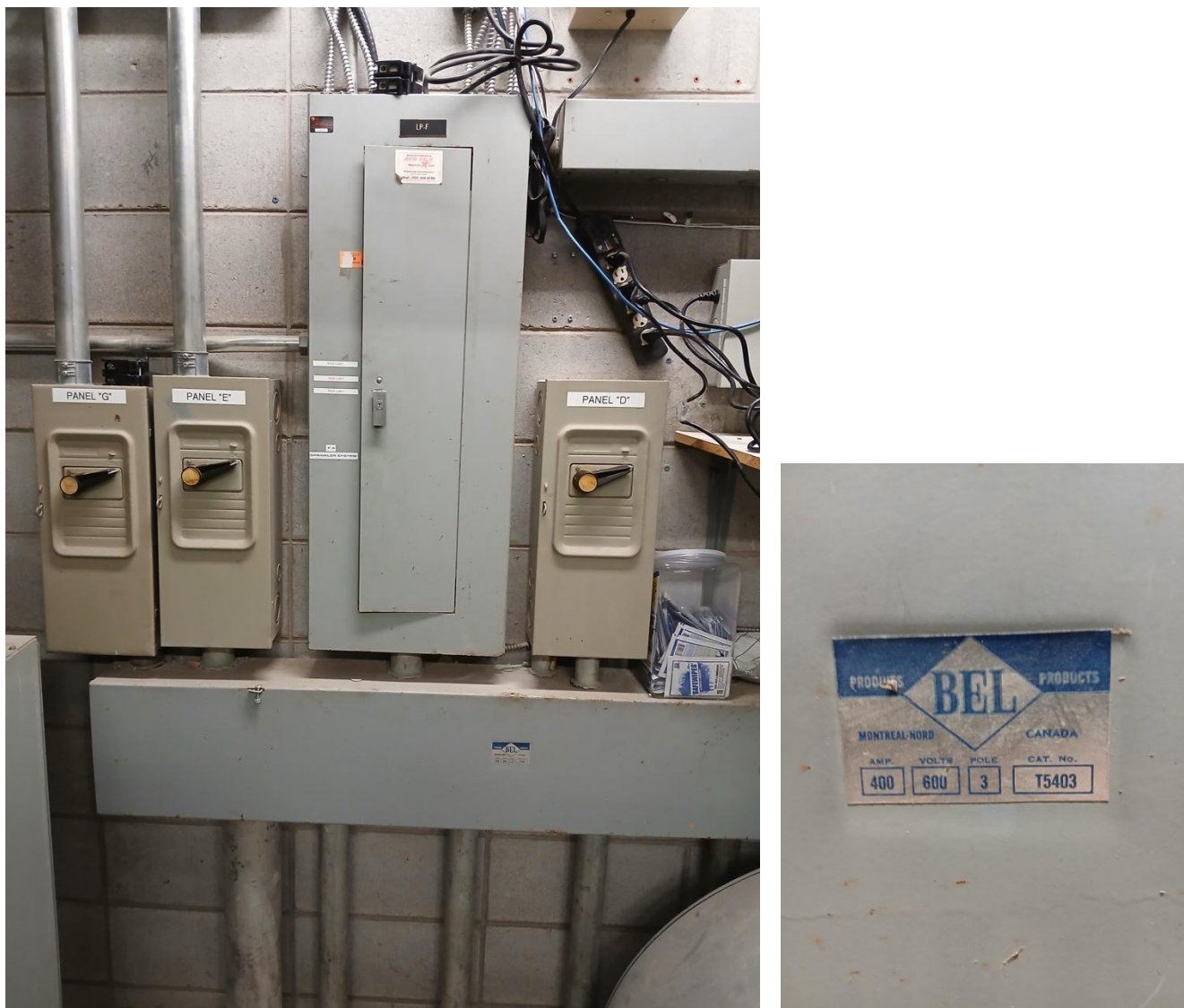
Figure 4-32: Photo taken by facilities staff of the splitter in the Electro-Mechanical room (left), along with the nameplate (right)
