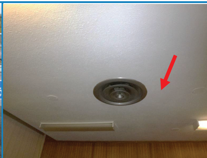
Photo 2: Typical view of the asbestos containing texture coat ceiling (see arrow) observed throughout the subject building.
