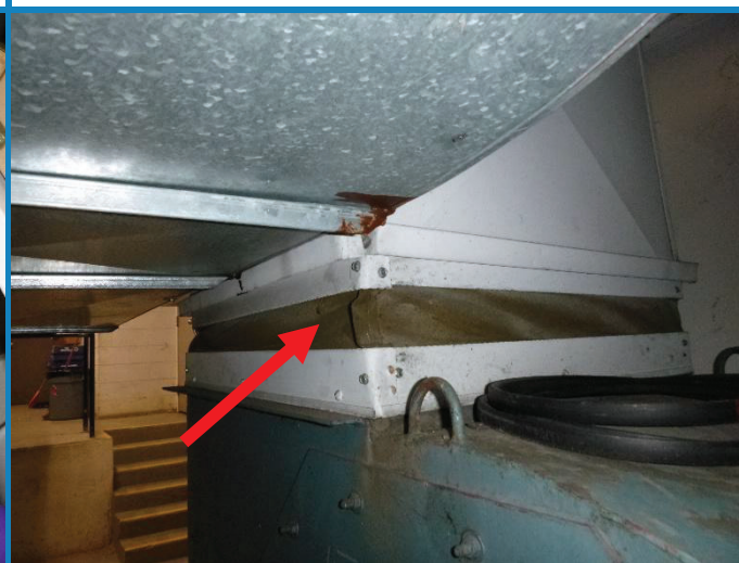
Photo 8: View of the presumed asbestos containing vibration dampers (see arrow) observed in the lower level boiler room.
