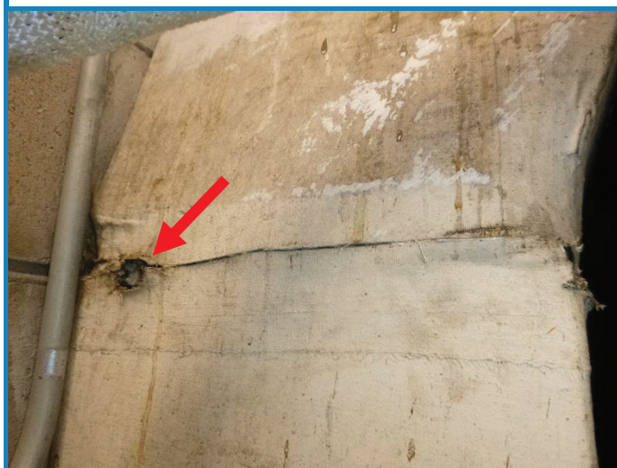
Photo 3: View of the damaged paring cement duct insulation (see arrow) observed within the penthouse Mechanical Room of the subject building.
