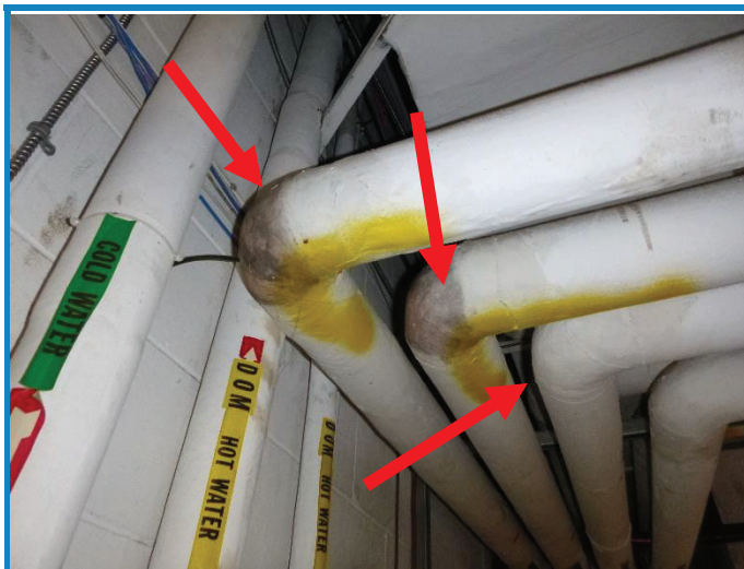
Photo 5: Typical view of asbestos containing paring cement insulation (see arrows) observed on pipe fittings observed throughout the subject building.
