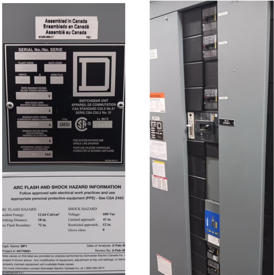
Figure 4-23: Photos of the switchboard nameplate (left) and distribution section (right) collected by NCC facilities staff
