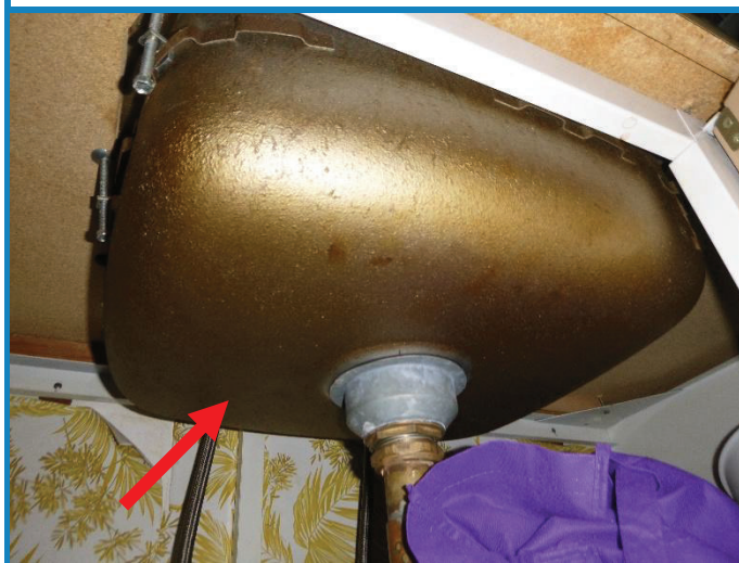
Photo 7: View of the gold anti-sweat mastic (see arrow) that is presumed to contain asbestos was newly observed underside of the kitchen sink of staff room in lower level of the subject building.
