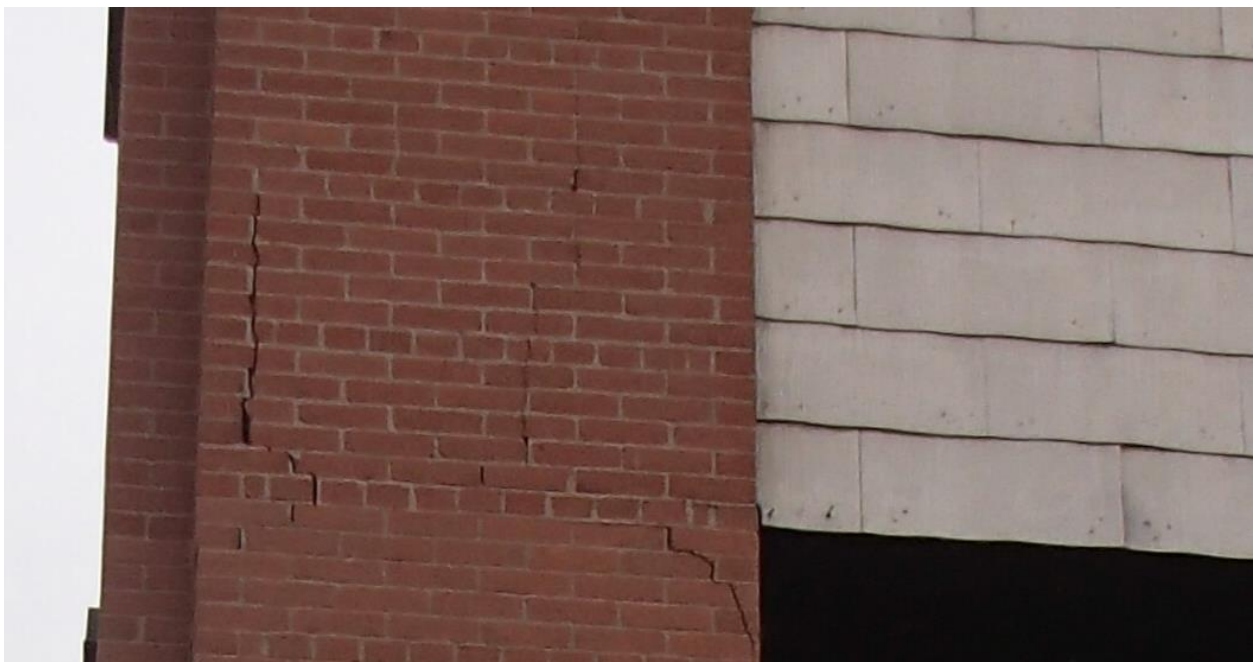
Crack in bricks - closeup
