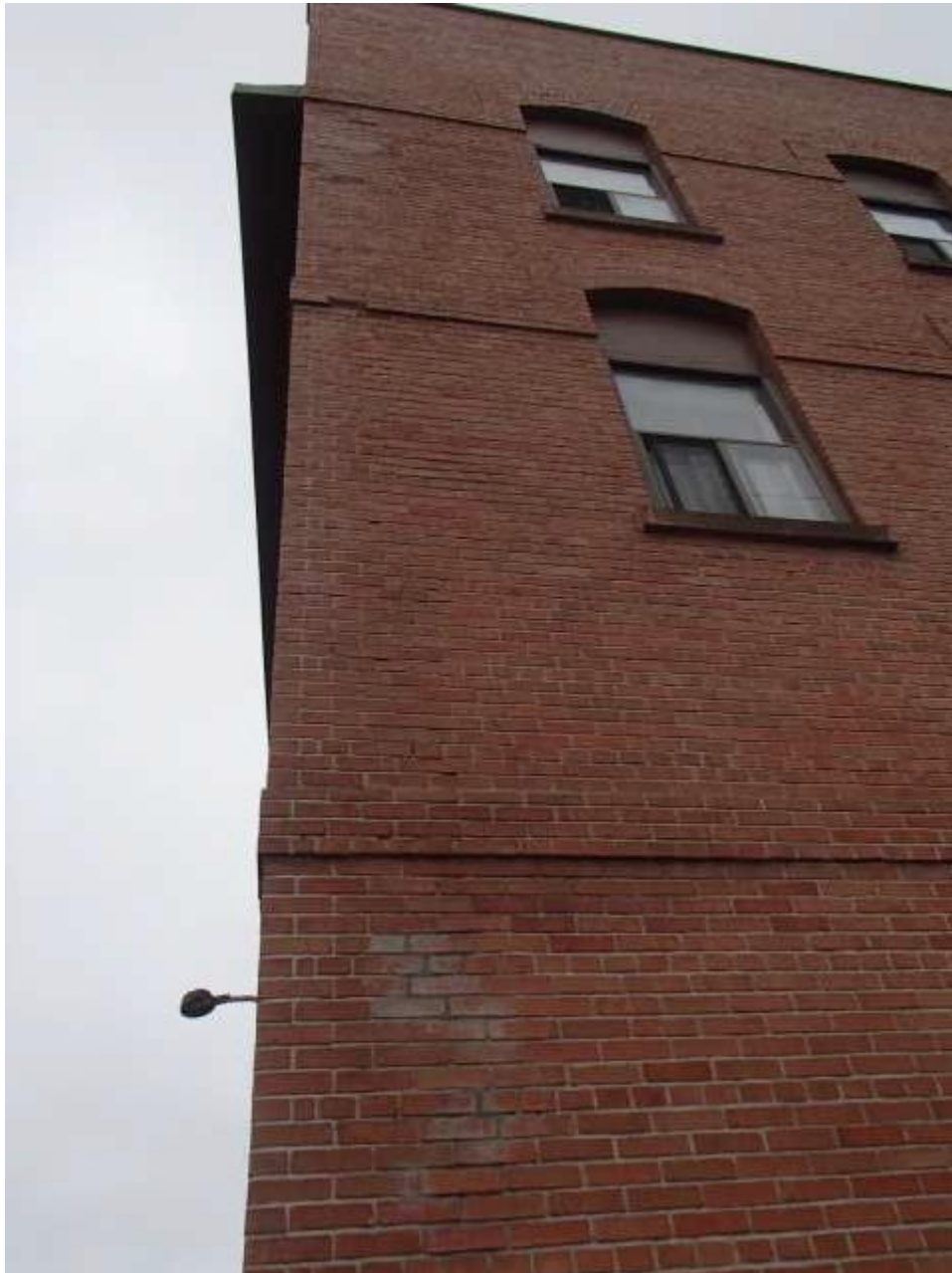
North wall - spalling
