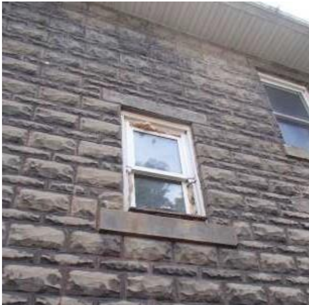
North side – window has insulation sticking out
