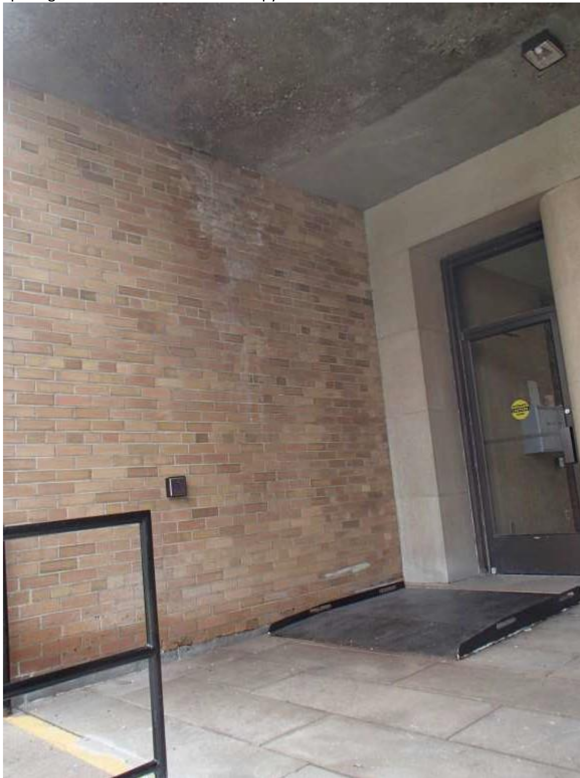
Spalling at front door – related to canopy
