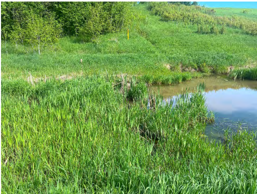
Photograph 4: View of eastern part of the Bennett-West Davignon Diversion Channel facing northward taken from northern boundary of the Subject Property.
