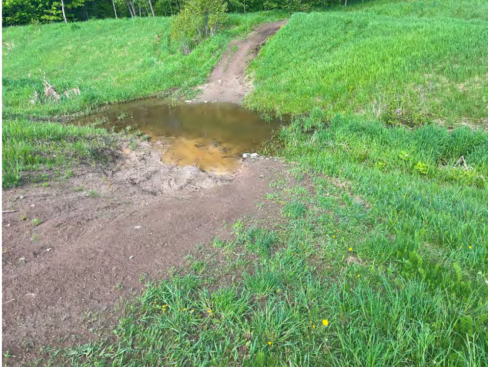
Photograph 5: View of ford across the Bennett-West Davignon Diversion Channel near the northeastern corner of the Subject Property facing northwestward.
