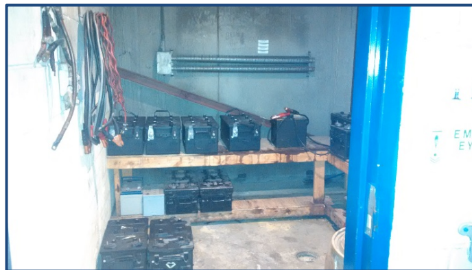
Battery Storage Room
