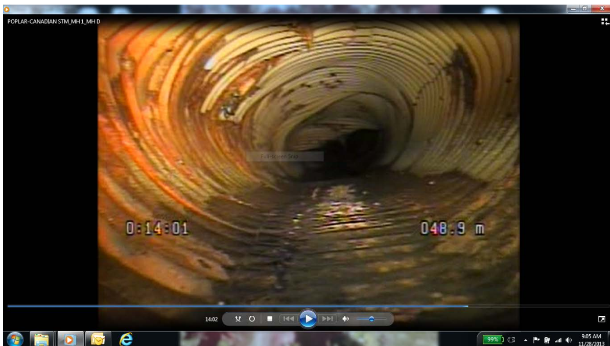
450 mm storm sewer draining west from Poplar Avenue through Canadian Motor Hotel parking lot
