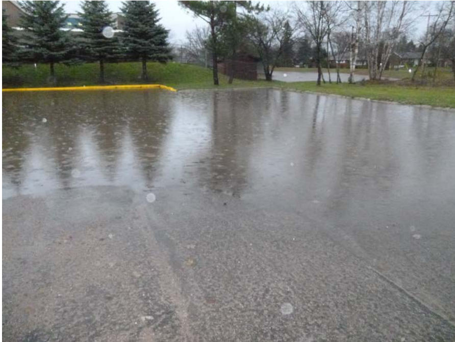
Ponding in parking lot of 205 McNabb Street Nov 17/13
