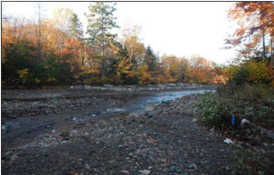
Photo 54. Erosion at Canon Creek, Area I.
